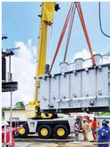
Employees from Distribution East offload the new 66 kV transformer during the project to upgrade the Santa Rosa 66 kV Substation in March.
